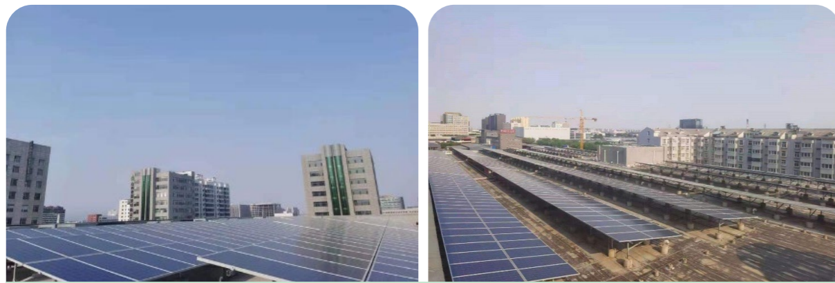
Rooftop photovoltaics equipment of Sinopharm Shanxi
