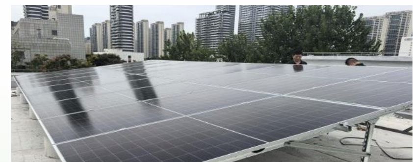
Photovoltaic Power Generation at Zhonglian Pharmaceutical
